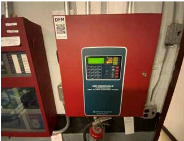
39 - FIRE ALARM PANEL
